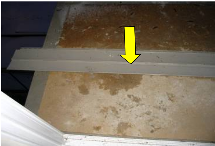
Photo 1: This photo shows the siding hanging over the unguarded end of the balcony. The arrow indicates the pencil line along the length three inches from the edge.
