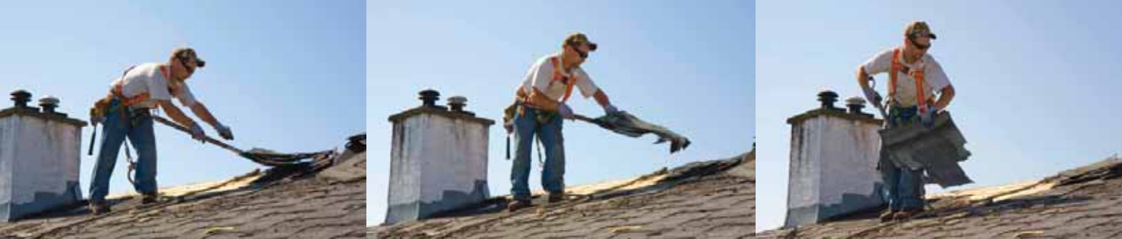
Nate Nelson, crew foreman for Parker Johnston Industries, conducts a tear-off of old asphalt shingles on a sloped roof in Saanich, B.C.
