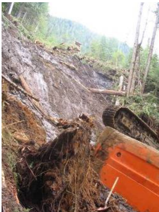
Photo 2: The excavator slid down a steep muddy slope and over a bluff.
