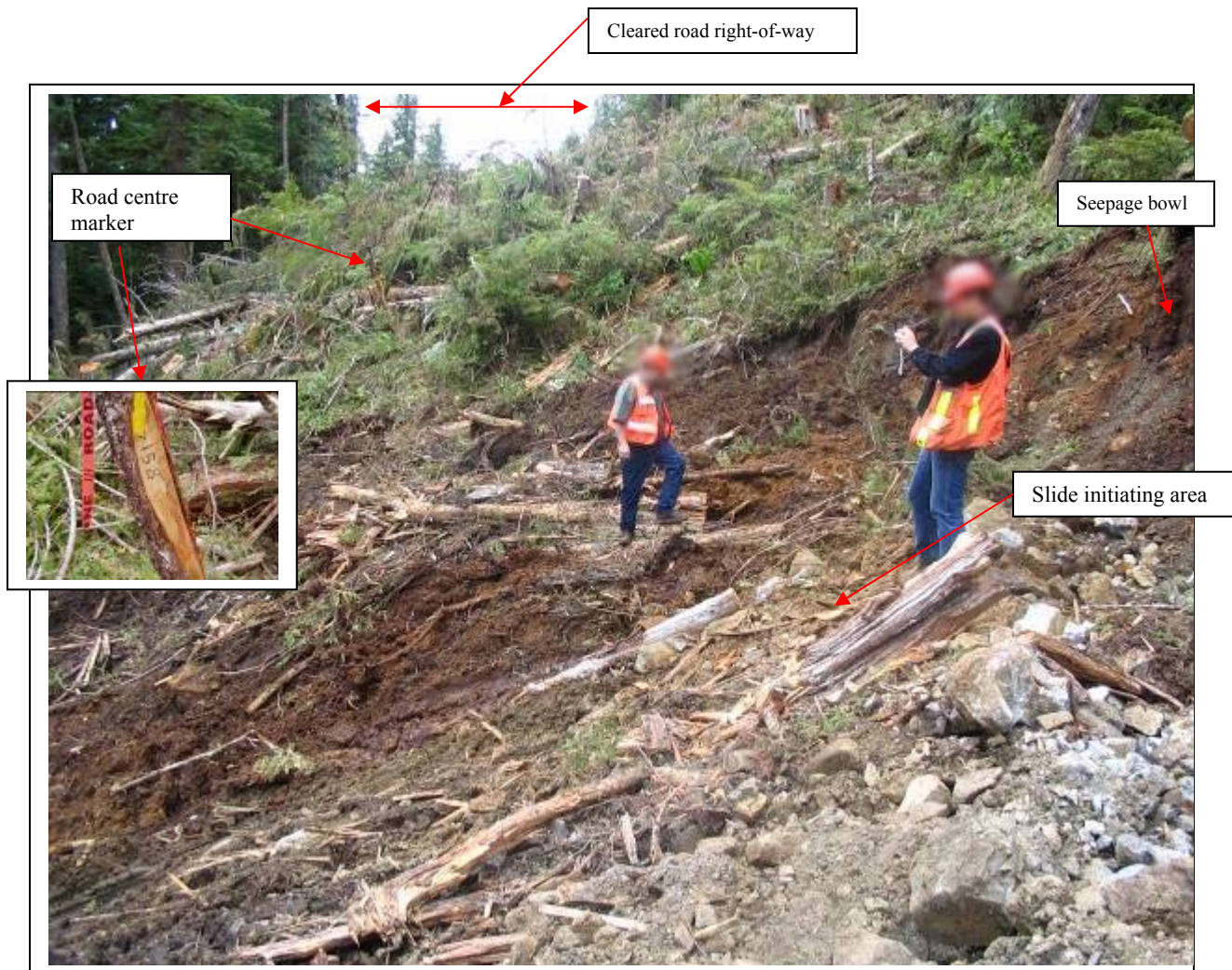
Photo 1: This photo taken after the incident shows the location of road centre marker.
