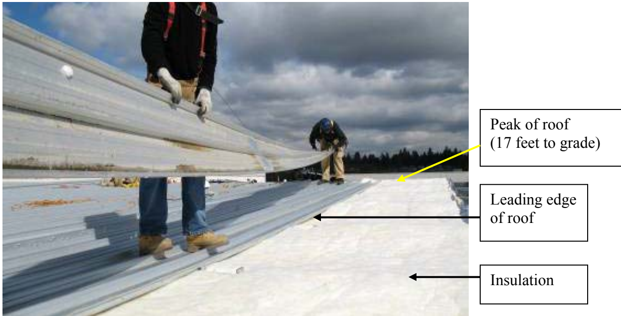
Figure 2: After the incident, workers (wearing fall protection) show how the roof panels were held as they were laid down.
