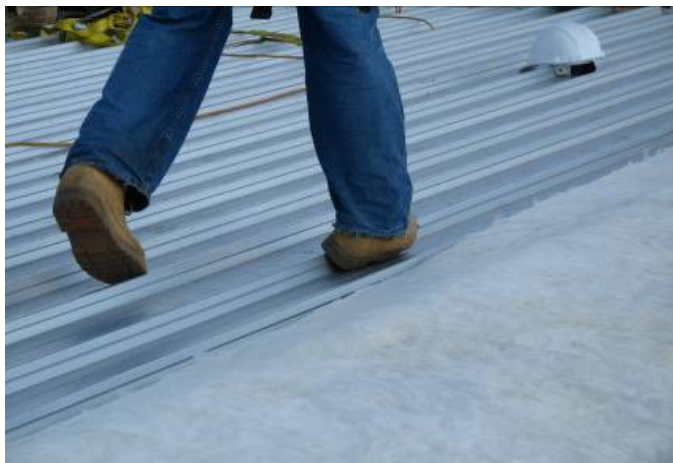
Figure 7: The protruding ribs form a tripping hazard.
