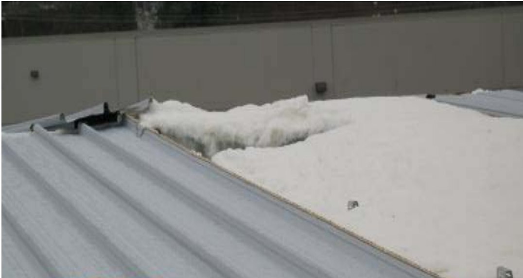
Figure 6: Close up view of the hole in the insulation where Worker 1 fell. The protruding ribs on the panel are visible.
