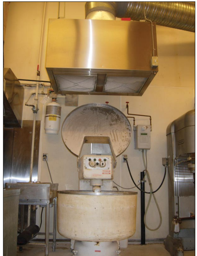
Dough mixer retrofitted with a cover and exhaust ventilation
